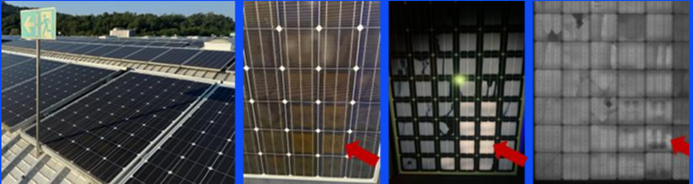
Figure 2: (a) Rooftop PV system exposed to persistent shading for more than 11 years; (b) encapsulant discolouration; (c) increased UV fluorescence indicating accelerated degradation; (d) corrosion visible in electroluminescence imaging.
